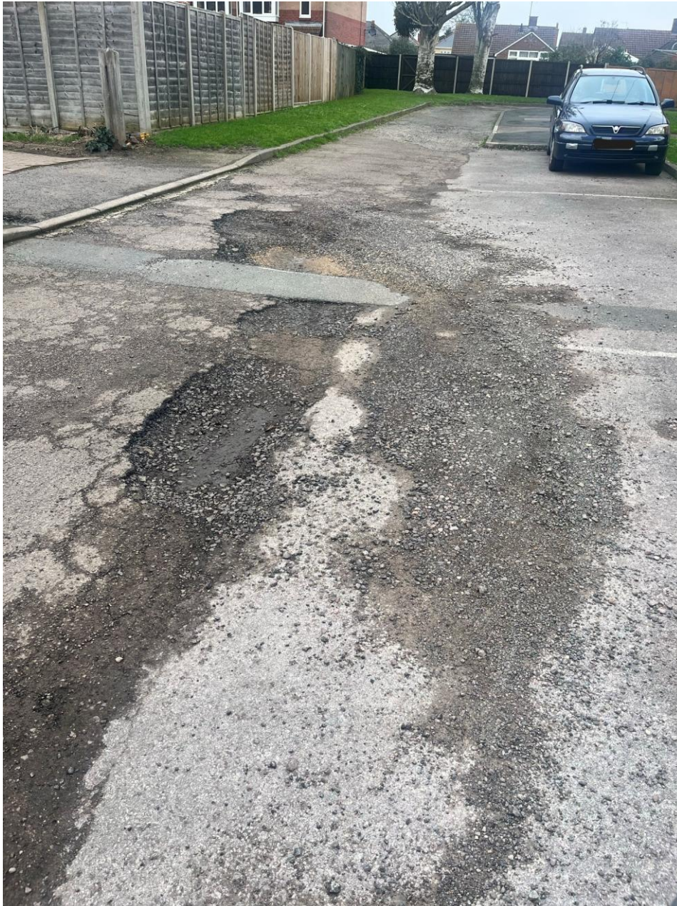
Victoria Court access road condition
